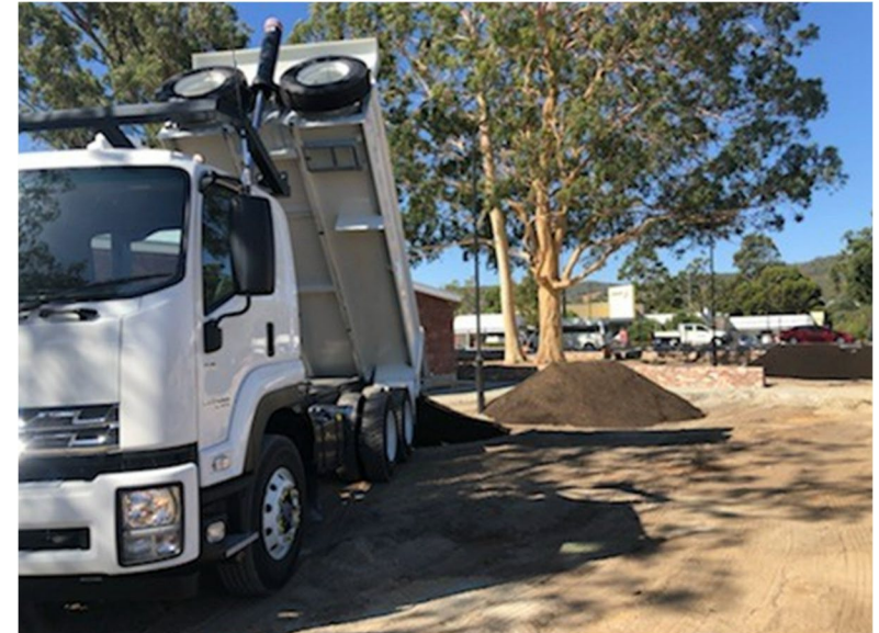
Above: A truck delivers FOGO material to the METRONET Denny Avenue Level Crossing Removal project
