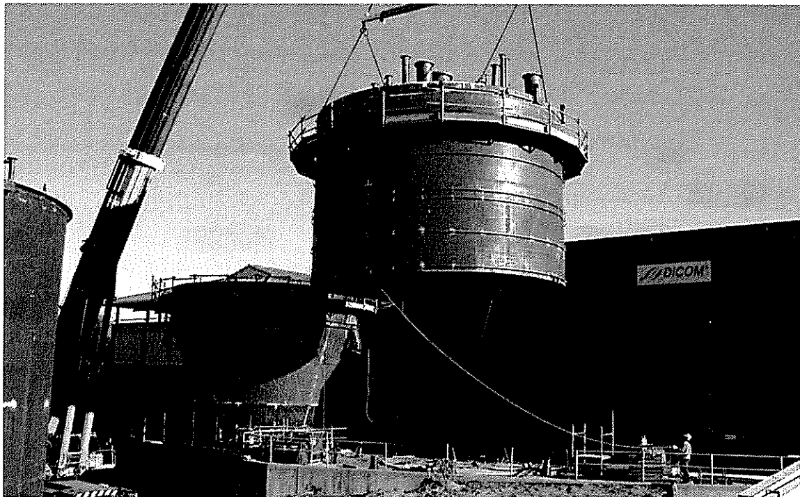
3. Upper part of DiCOM vessel with top section in place, being lifted onto lower part.
