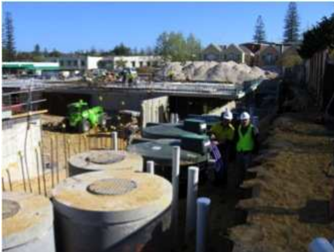
Figure 5 - Photo of installation of wastewater recycling system at the Cottesloe - Peppermint Grove - Mosman Park Combined Library (Source: http://thegroveprecinct.com/the-building/water-systems/#wastewater ).
