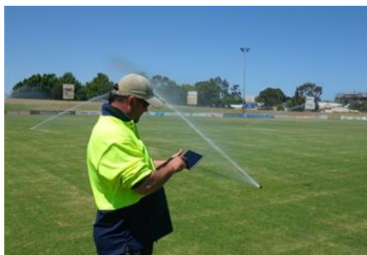
The Town of Bassendean's irrigation control system enables staff, at the touch of a button, to reset irrigation schedules and turn off sprinklers when rain is due Photo: Town of Bassendean
