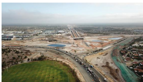
The Tonkin/Reid intersection under construction: road infrastructure is a priority for Perth's Eastern Region Photo: Main Roads WA
